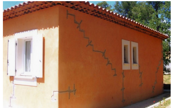
Fissuration de façades. © BRGM
