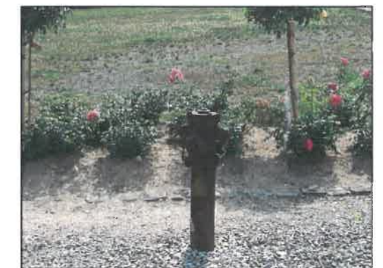
Poteau incendie Source TOPOS
