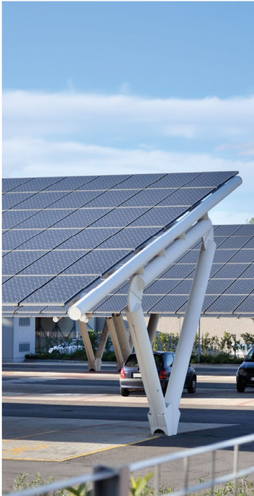
Parking couvert d'ombrières photovoltaïques
