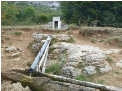
Absence clapet anti-intrusion
