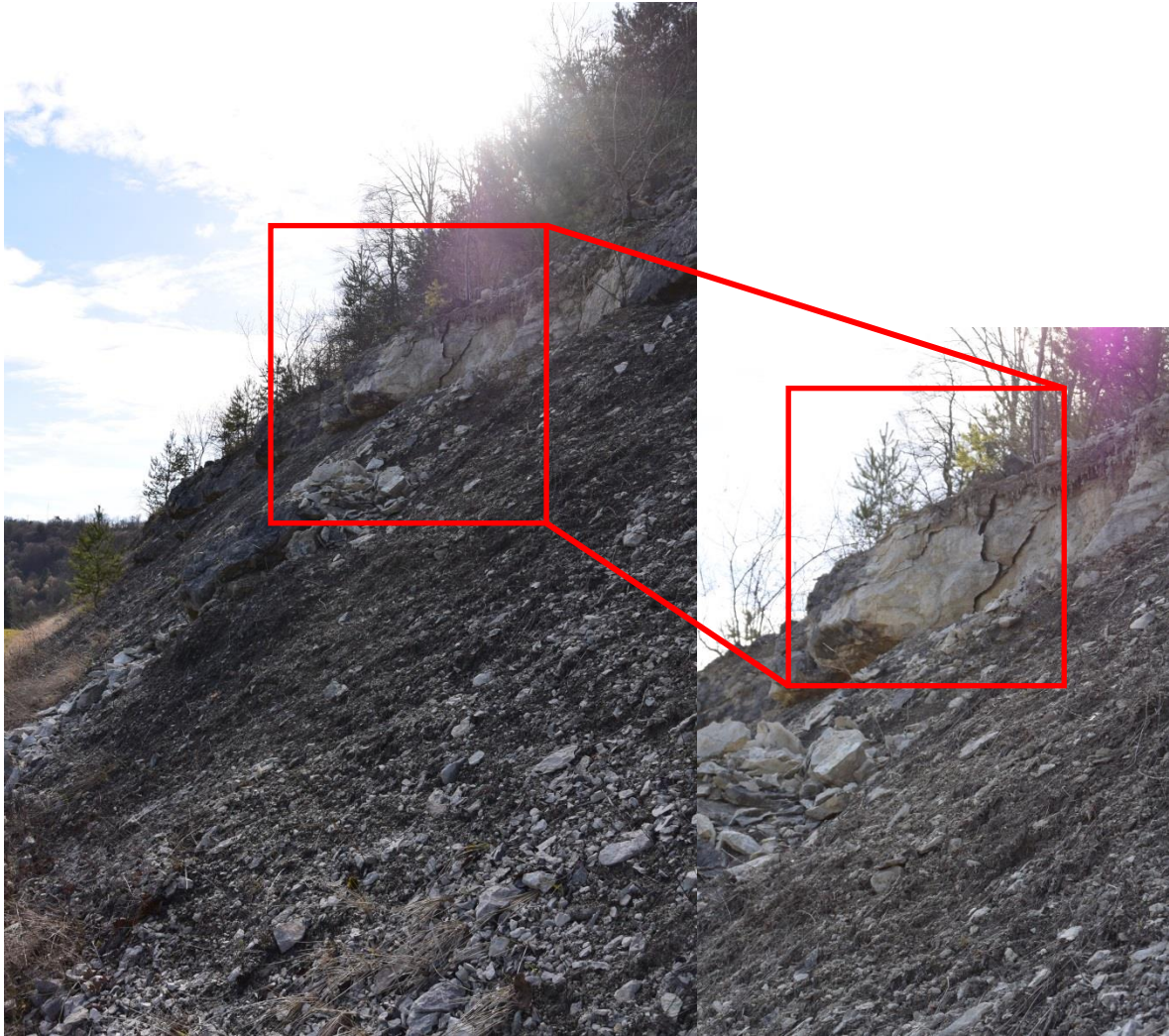
Illustration 11 – Eboulement rocheux imminent (mars 2015, BRGM)
