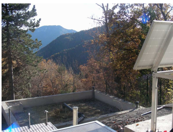
Photo 2.3.3.2. Station épuration Villeplane
