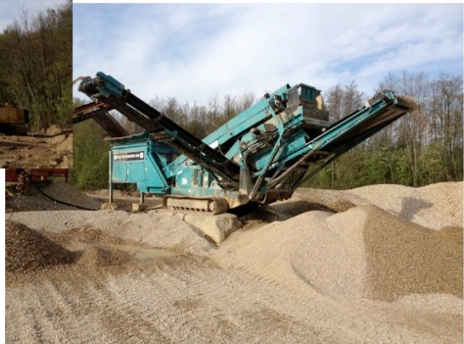
Installation de criblage
